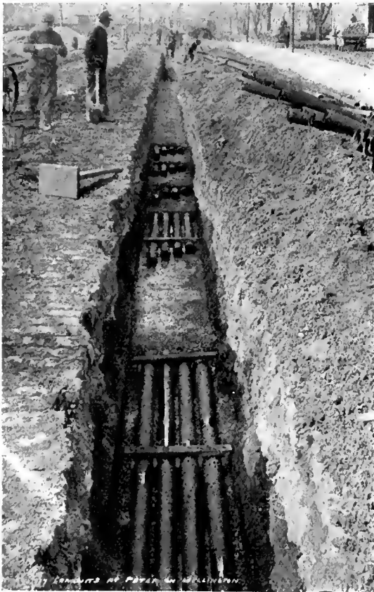
Fig. 1—24" fibre duct, 1 1/2" spacing between ducts.
